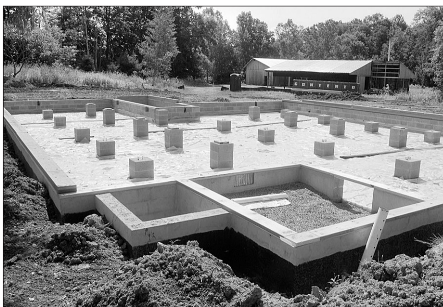
A recently built foundation awaits Lime Hollow's new education center building, which will be placed on the foundation later this summer.
